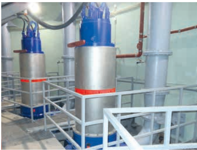
Main pumps Amarex KRT K 400-710
