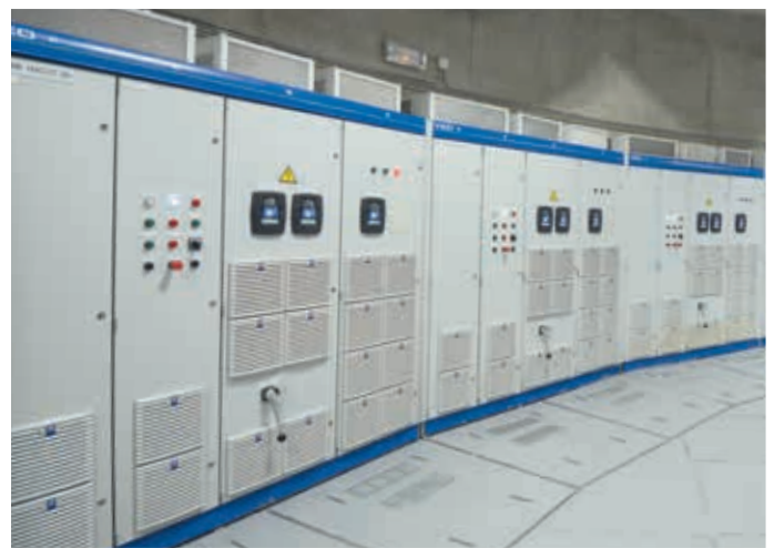
Control cabinets for control equipment
